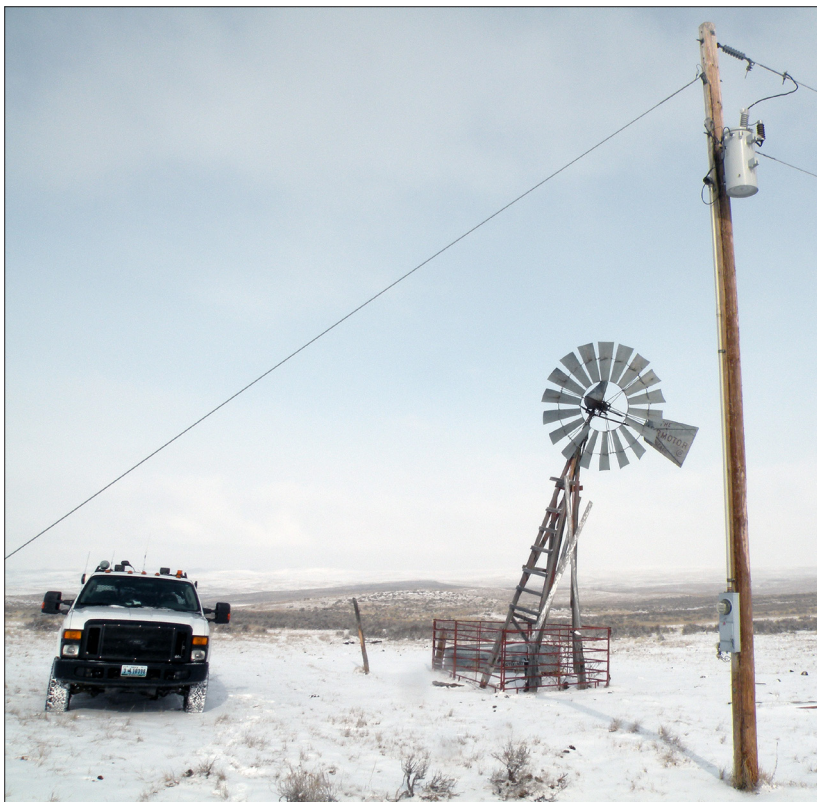
Photo by PRECorp Distribution Design Tech Luke Blakeman
